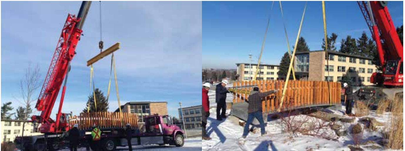
Fig. 5: The completed footbridges were transported on a flatbed truck and installed with a truck-mounted crane
